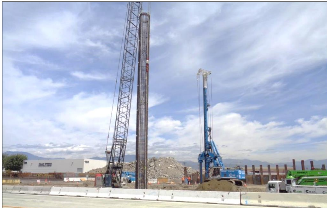
CAST IN DRILL HOLE PILE DRIVING – PUENTE AVENUE GRADE SEPARATION PROJECT – CITY OF INDUSTRY
